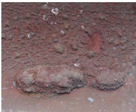
Figure 4. The inner surface of the nearby piping of flaw state samples
